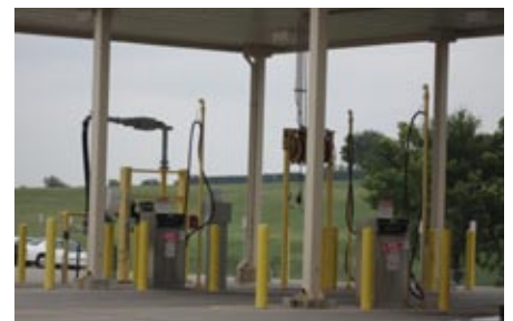
Gas station pumps at the new Fort Worth Service Center
