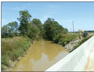
Figure 2. A project participant installs a drop pipe structure, which will allow the discharge runoff water to empty directly into Bayou DeVew rather than drain across an erosion-prone field.
