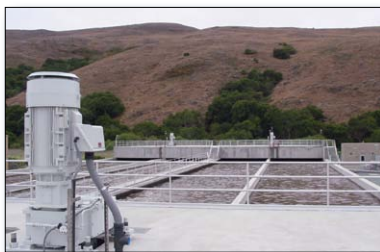
Figure 4. Building this new wastewater treatment plant helped remove point source discharges from Chorro Creek.
