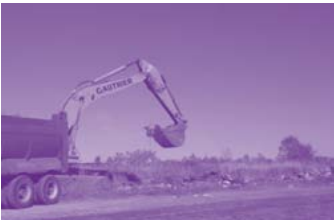
Oneida's reclamation equipment.
