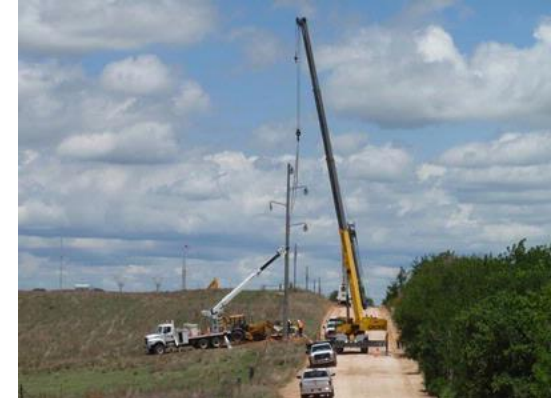
Seven miles of transmission lines
