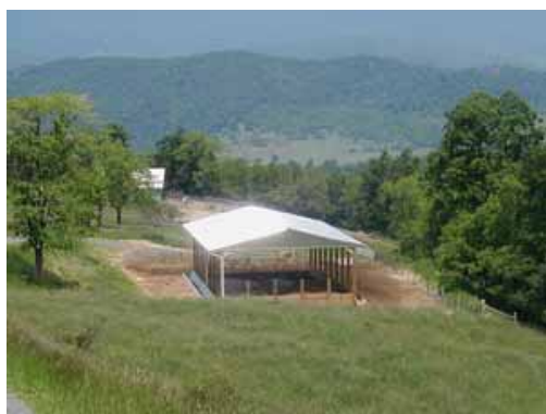
Animal feeding area after installation of waste storage facility, runoff control system, stream fencing, clean water diversion, paved feeding area, livestock watering facility, stabilized access road, and critical area planting.
