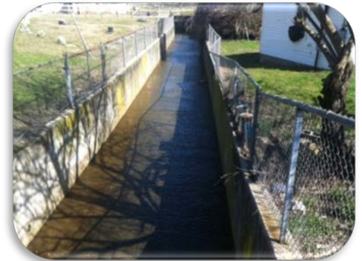
Watts Branch near Davey St. Much of the stream is in concrete channels/culverts.
