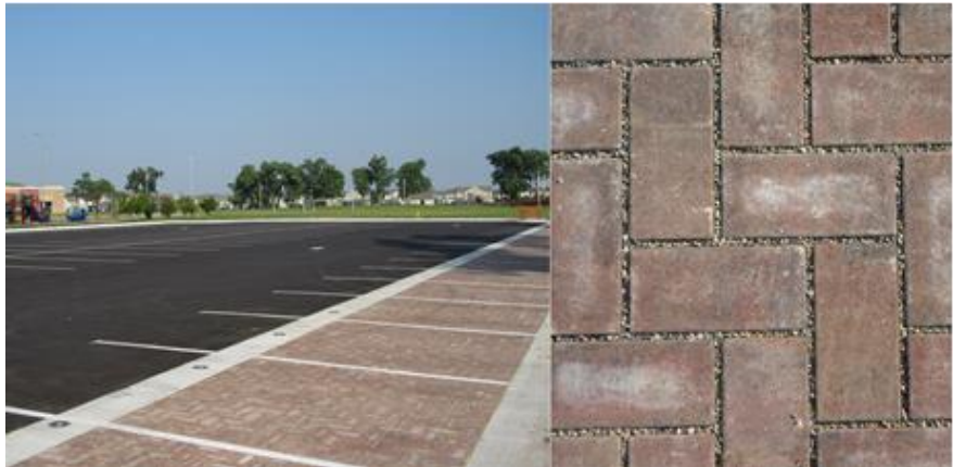
Left: The completed permeable pavement parking lot behind Seitz Elementary School on Fort Riley. Right: When it rains, stormwater infiltrates through the gravel-filled spaces between these pavers into the ground below.
