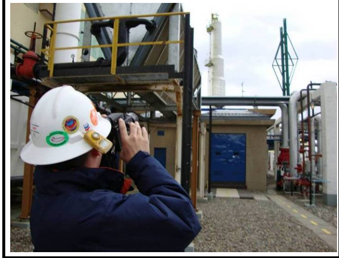
Exhibit 2 A measurement expert uses the GasFindIR Camera to survey the Posesión Plant.
