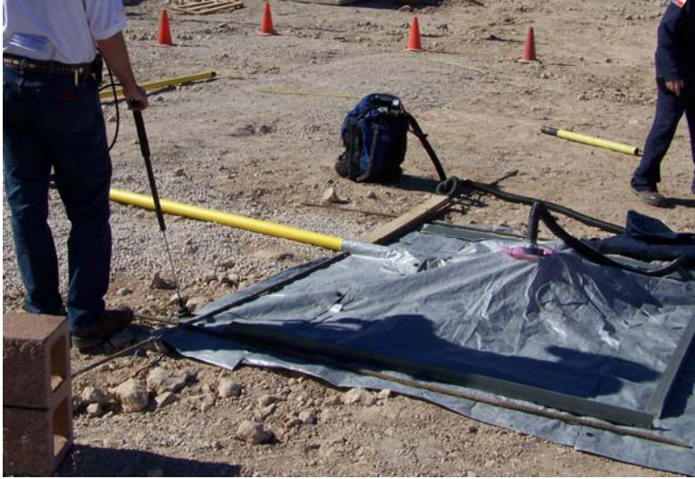
As part of a GTI study, Southwest Gas conducted a surface measurement of methane flow-rates from an array of custom-built underground pipes.
