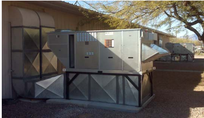
A newly developed high efficiency natural gas heat pump, shown here at Davis Monthan Air Force Base, is now available for commercial applications.
