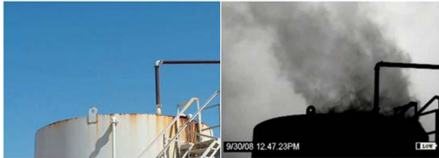
Methane Leaks from Storage Tanks
