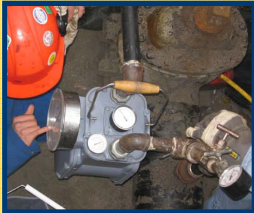
Exhibit 1: Diaphragm meter deployed to measure leak rate of an isolated length of Enbridge’s cast iron pipe.
